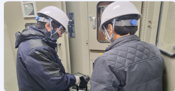
Safety Inspection of Electrical Facilities at Naju Building
